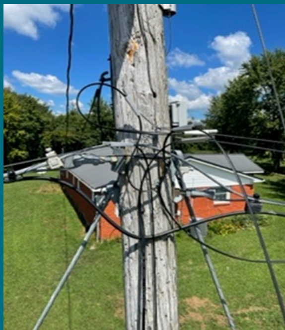
What a mess the contractor made connecting drops on a pole.
